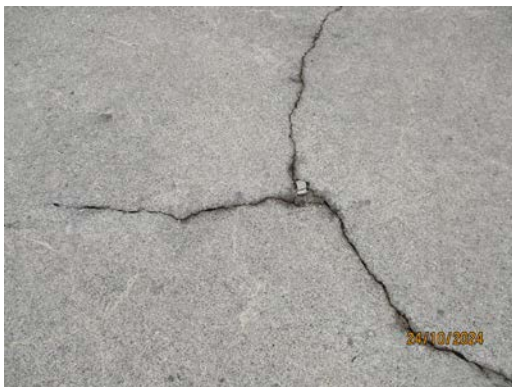
Roof top “spider crack”
