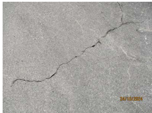
Typical roof topside crack
