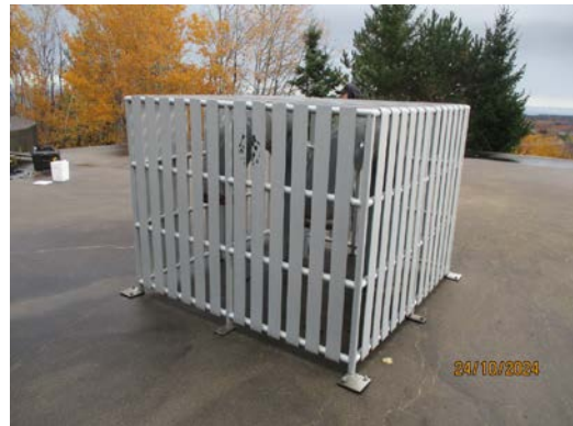
Protective cage around two gooseneck vents
