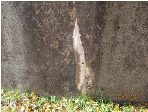
*Close up view: Typical cracking
