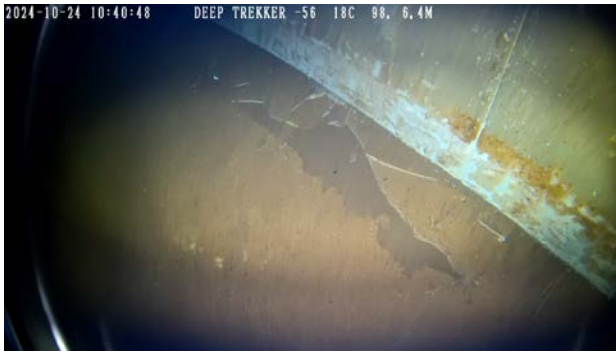
Outer floor, parging layer flaked off
