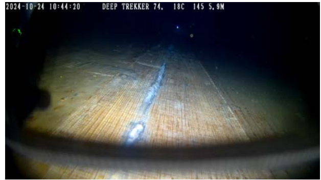
View up wall joint; white deposits coming through
