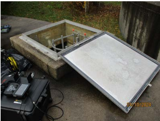
Manway cover; rubber seal in good condition
