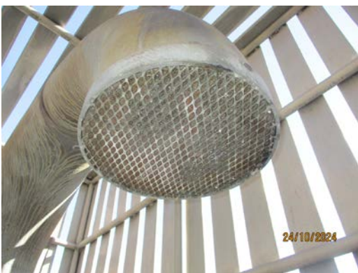
Vent one of two, screening is ok
