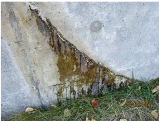
View of wet deposits from concrete layer
