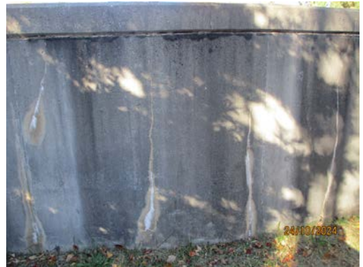
Example of multiple cracks with white deposits
