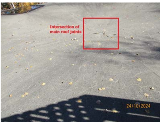
Typical white deposits
