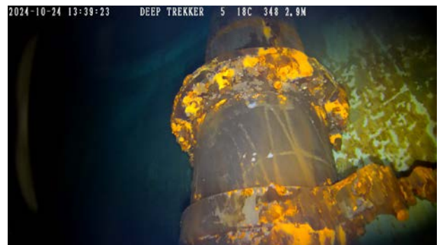
Scale and deposits on overflow piping & bracket
