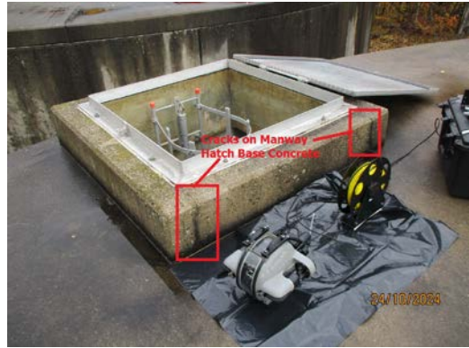
Concrete base for roof manway; two cracks marked
