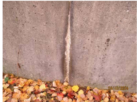
Typical area of white deposits at joint
