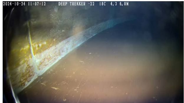
Wide view of wall to floor joint
