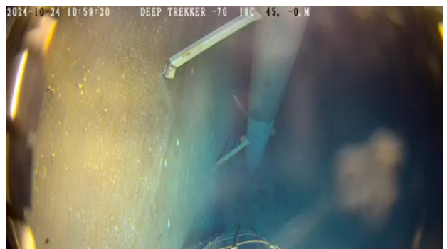
View stainless steel pipe and brackets
