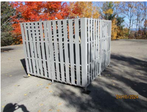
Protective cage around roof vent piping
