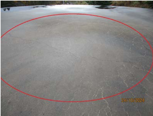
Roof top cracks around centre support area
