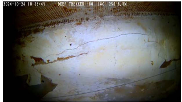
Cleared sediment away; cracked parging underneath
