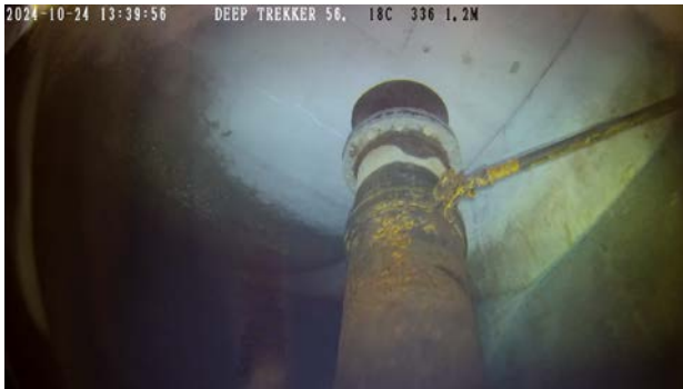
Upper portion of overflow pipe and bracket
