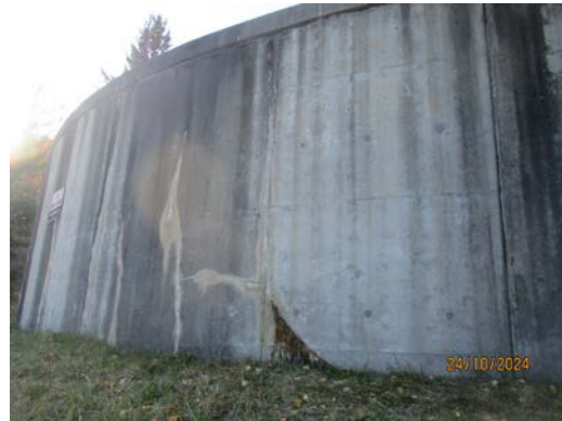
Wide view of area where wet deposits are seen
