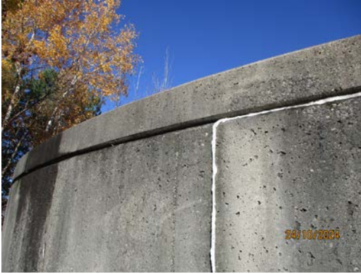
Grouting missing - external roof-wall joint
