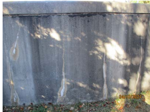
Example of multiple cracks with white deposits
