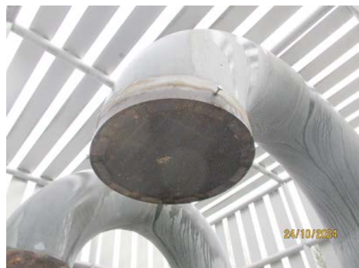
Underside of 2 nd gooseneck vent screen – ok
