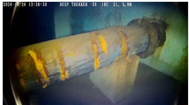
Fill pipe to wall interface, scale deposits on pipe
