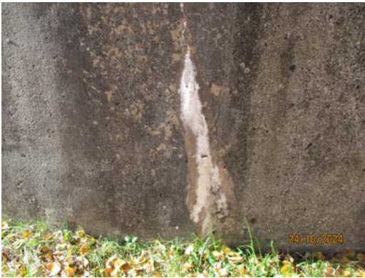
*Close up view: Typical cracking
