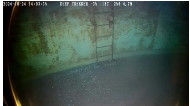
Ladder bottom, bits of scale laying loose on floor
