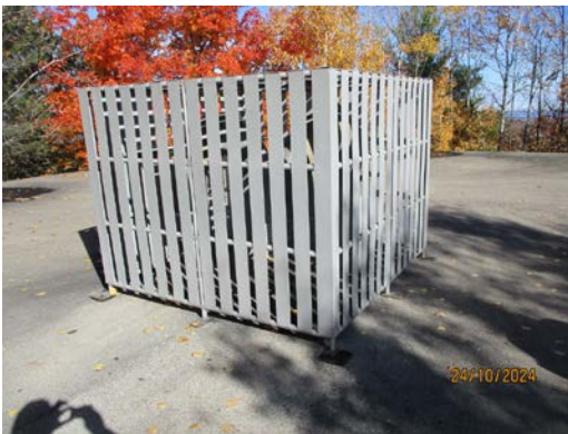
Protective cage around roof vent piping
