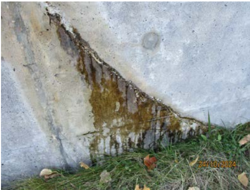
View of wet deposits from concrete layer
