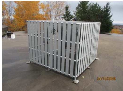
Protective cage around two gooseneck vents
