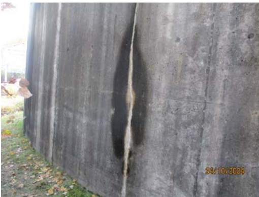
Example of crack indication with white deposits
