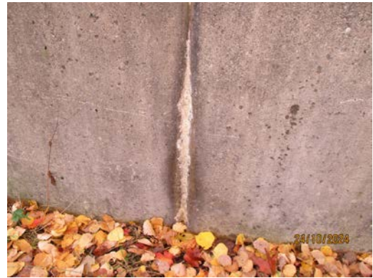
Typical area of white deposits at joint
