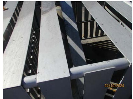
One strap on top of protective cage is bent inward
